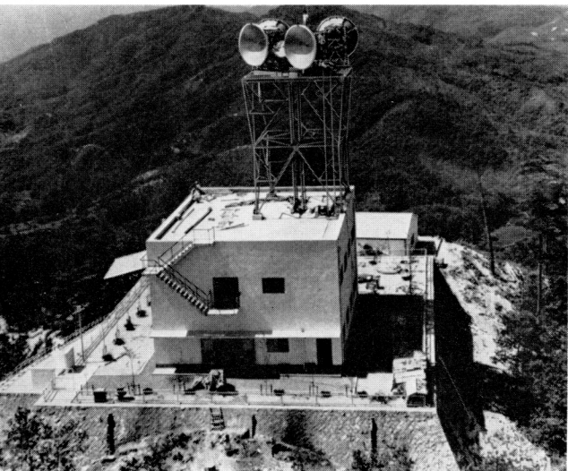
Back-to-back terminal equipment at Koi, Japan, part of a television and telephone microwave link
